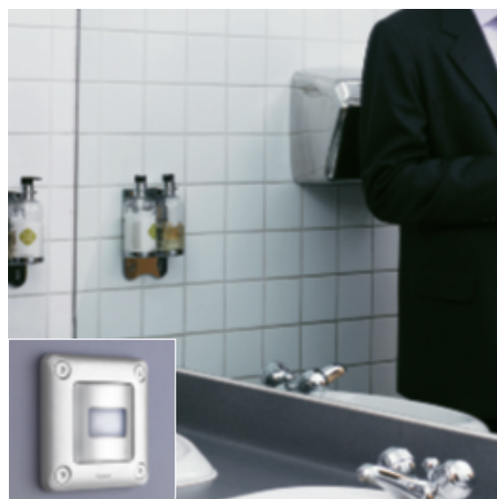
PUBLIC WASHROOMS | Automatic switch
